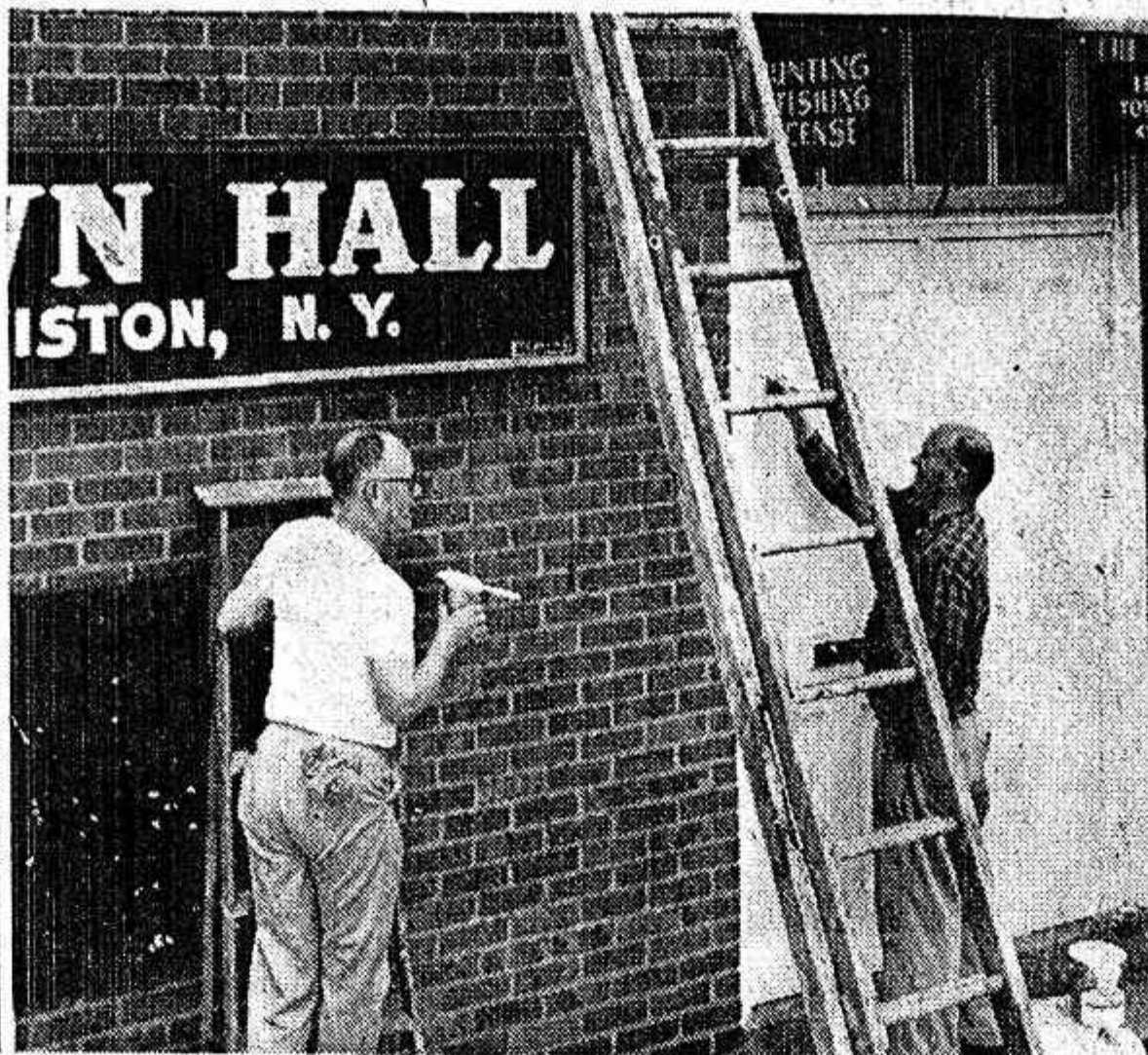
cleanup whirlwind. Mrs. Olaf Erickson, left, and Mrs. Paul Schmoyer, in photo at left, plant a floral tree in Center Street. In center photo, Ashton Wipple, left, and Arthur Kelly freshen up
